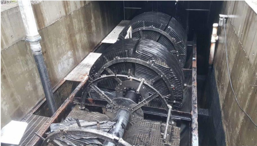
Photo 1:- View of Existing RBC with broken Media Pack 1.
