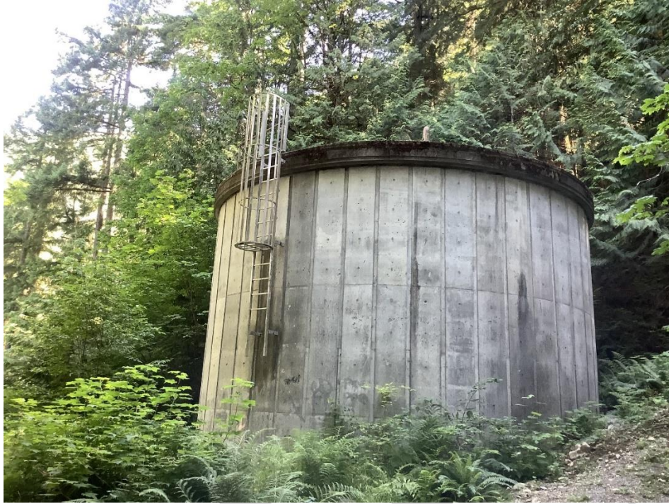
Photo 6. Five water storage facilities are found in the forest interface above the community.
