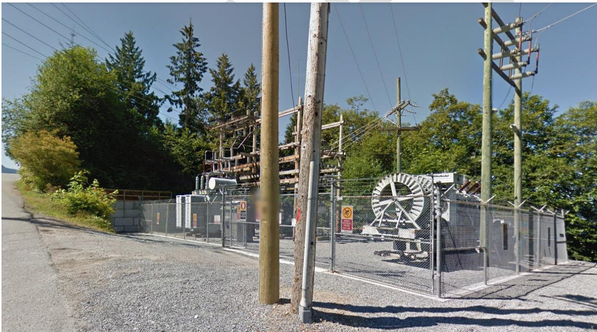
Photo 4. BC Hydro substation on Tidewater Road (Google Earth image)
