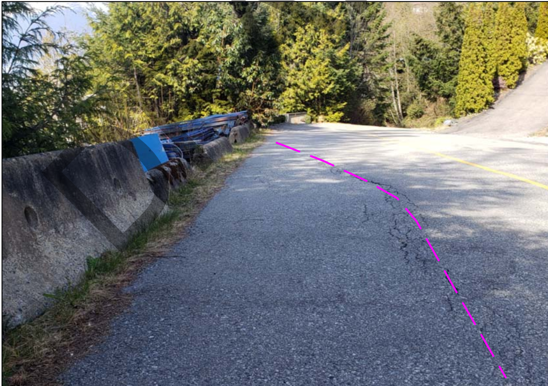
Photograph 7: view looking north showing cracked pavement beside slope crest.
