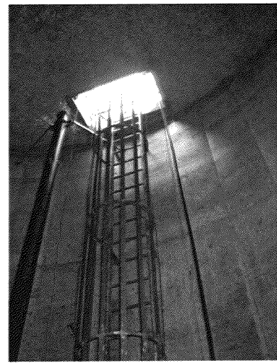
155. Access hole in of slab
