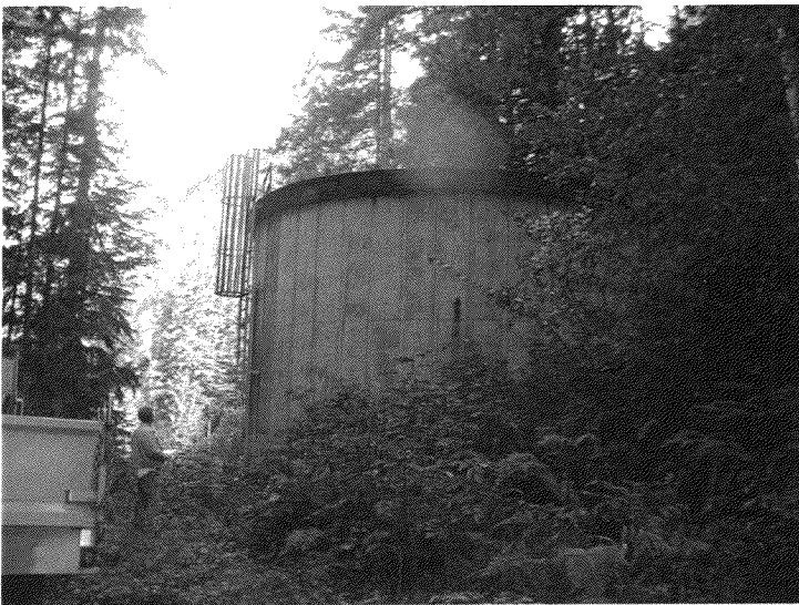
64. General view of tank
