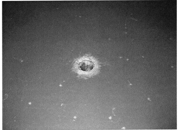
157. Dirt and grime at bottom of tank and at drain
