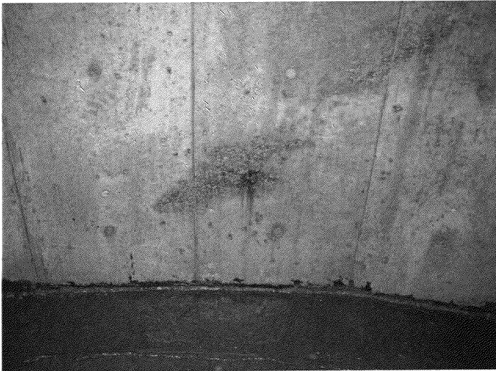
162. Small area of honeycombed concrete and stains from an exposed corroded rebar
