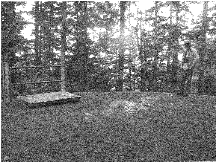
67. Debris/vegetation/algae on roof
