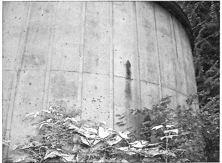
65. Evidence of honeycombed concrete on wall
