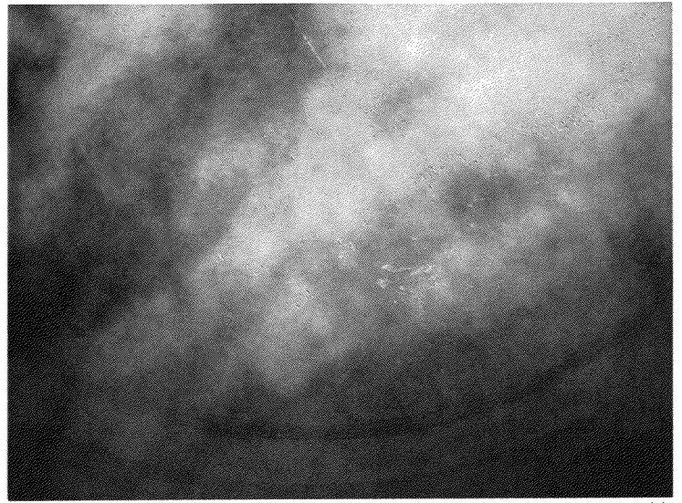
161. Tank roof from the inside. Note signs of florescence on the underside of the roof slab
