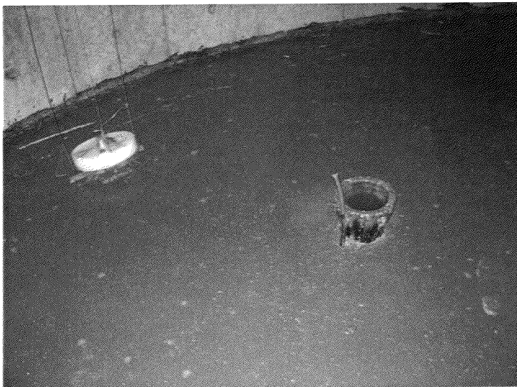
158. Level transducer to the left and inlet pipe
