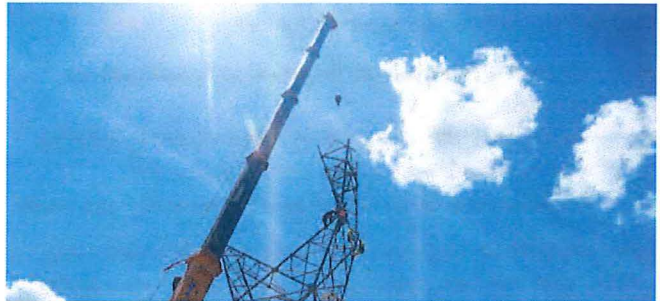
The project includes construction of more than 600 steel transmission towers with an average height of 42.5 meters.
