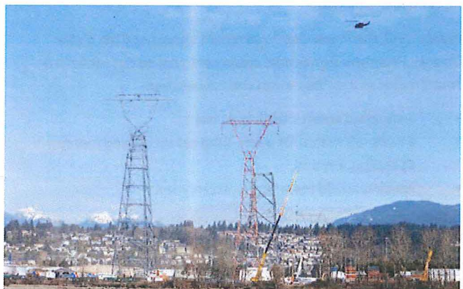
A helicopter was used to string transmission lines during the final phase of the Fraser River Towers restoration project.
