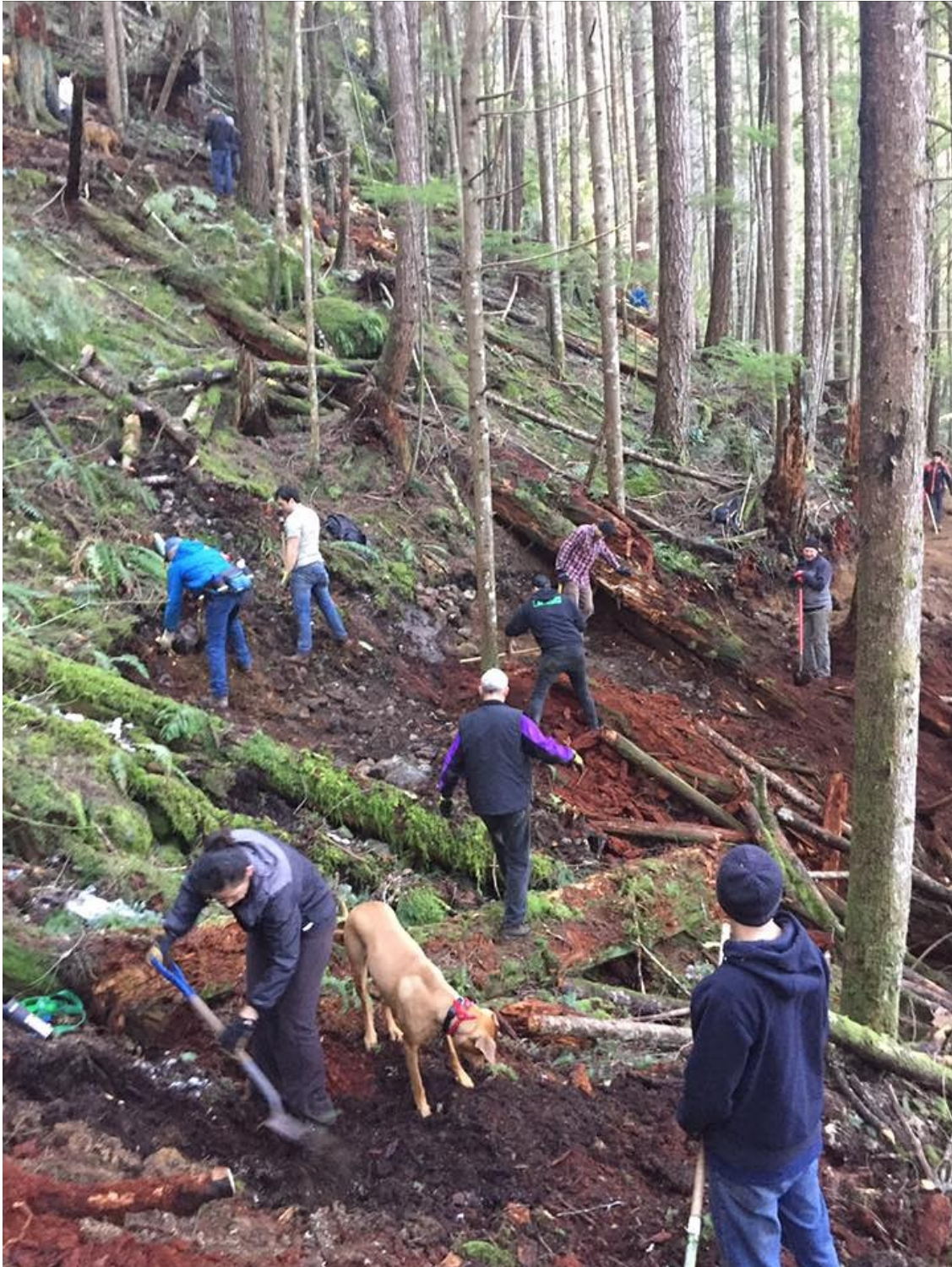
Great trail work participation from volunteers (70 – 80 diggers and dirt movers) with the Squamish Off-Road Cycling Association (SORCA) who made good progress on 500
