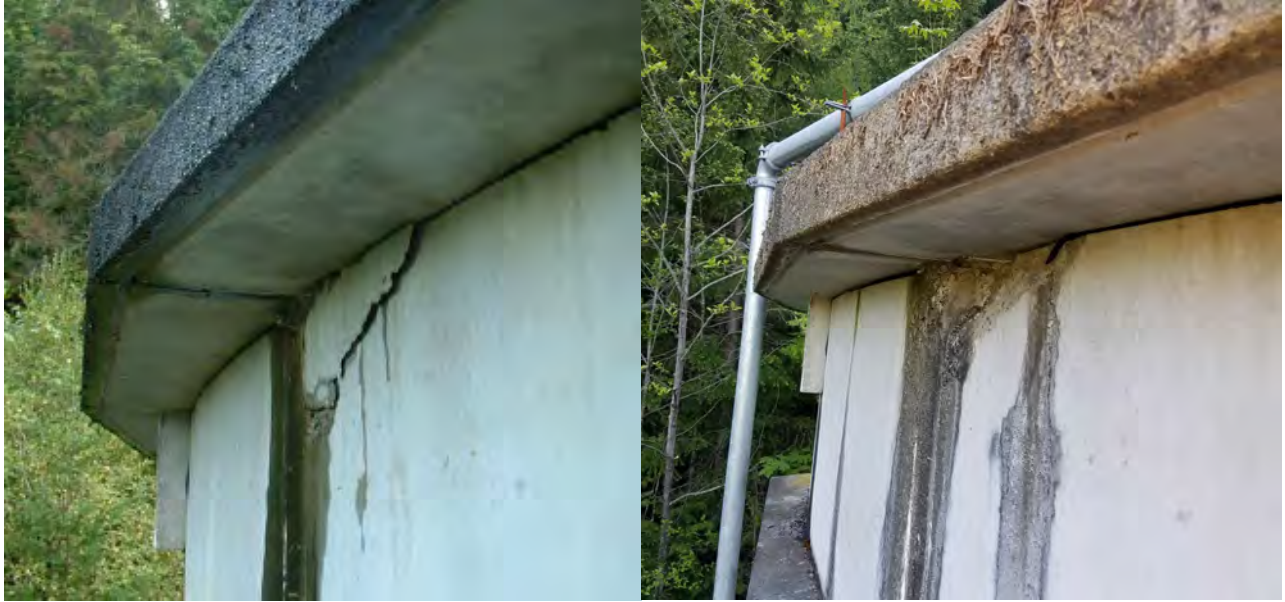
Figure A2.2.5: Wall/roof connection damage on north panels, left picture from 2005, right picture from 2018
