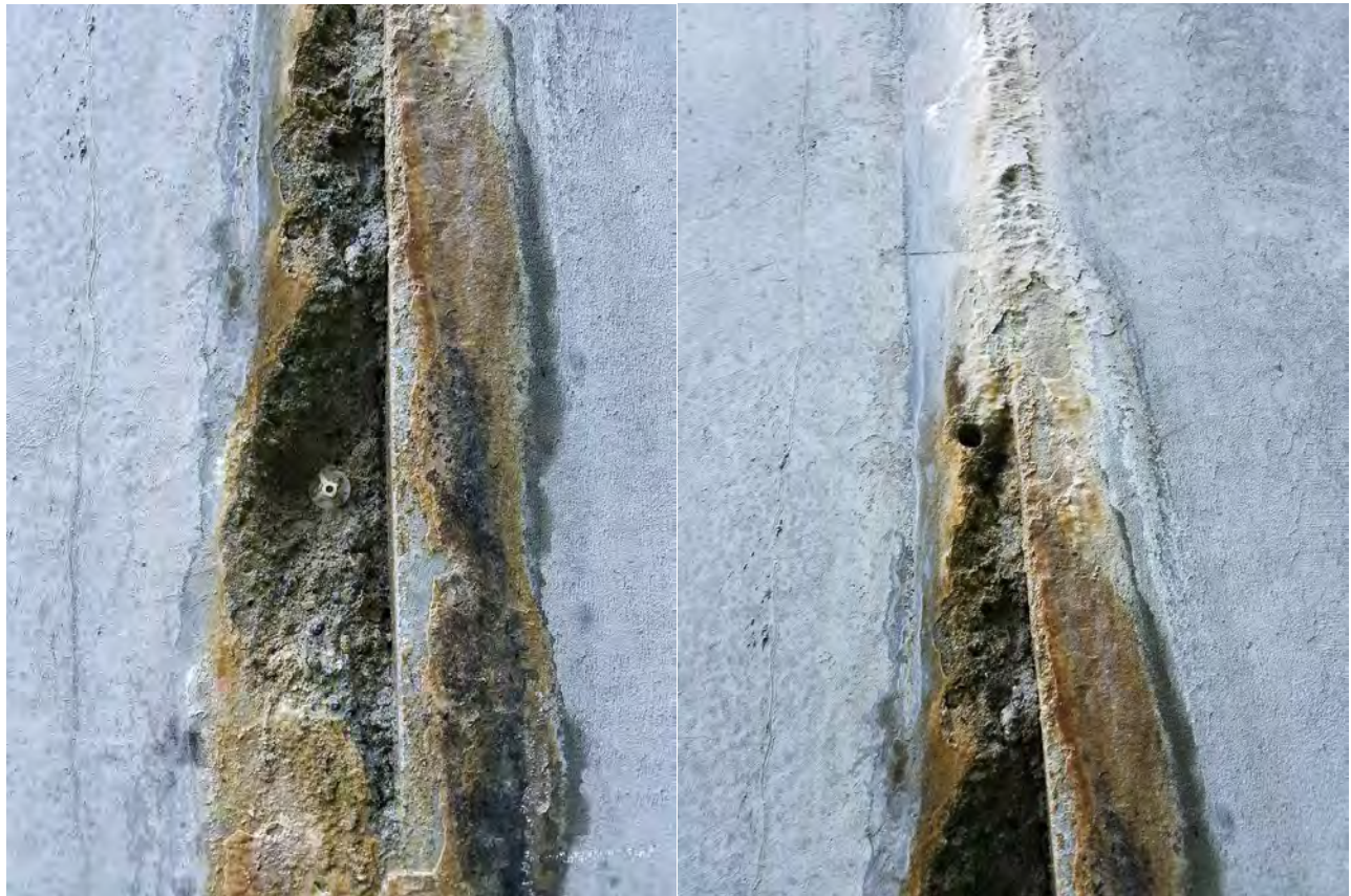
Figure A2.1.4: Wall panel material deterioration and evidence from previous repairs
