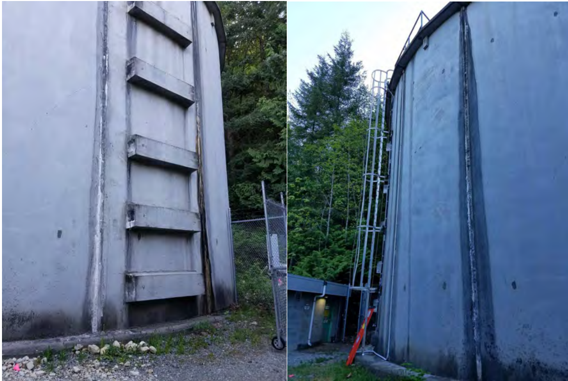
Figure A2.1.1: Wall panel leakage facing southwest (left) and northwest (right)
