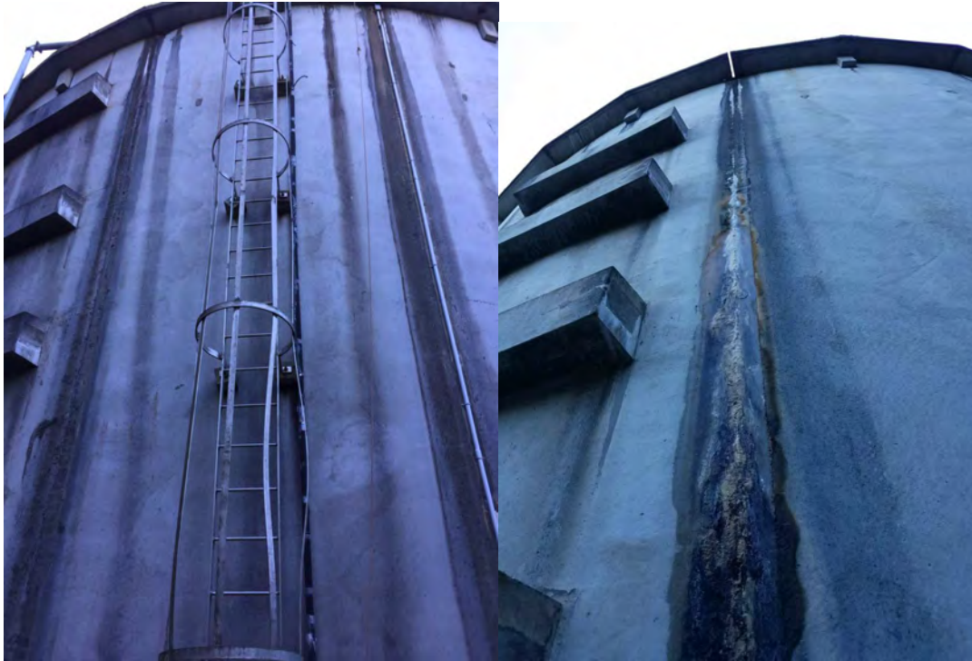
Figure A2.1.3: External access ladder cage (left) and wall panel leakage (right)
