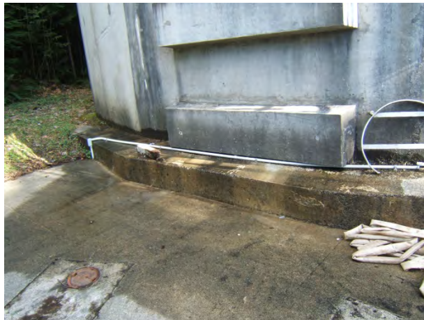
Figure 1: Record Photo of Horizontal Seam Leakage (March 20, 2006)
