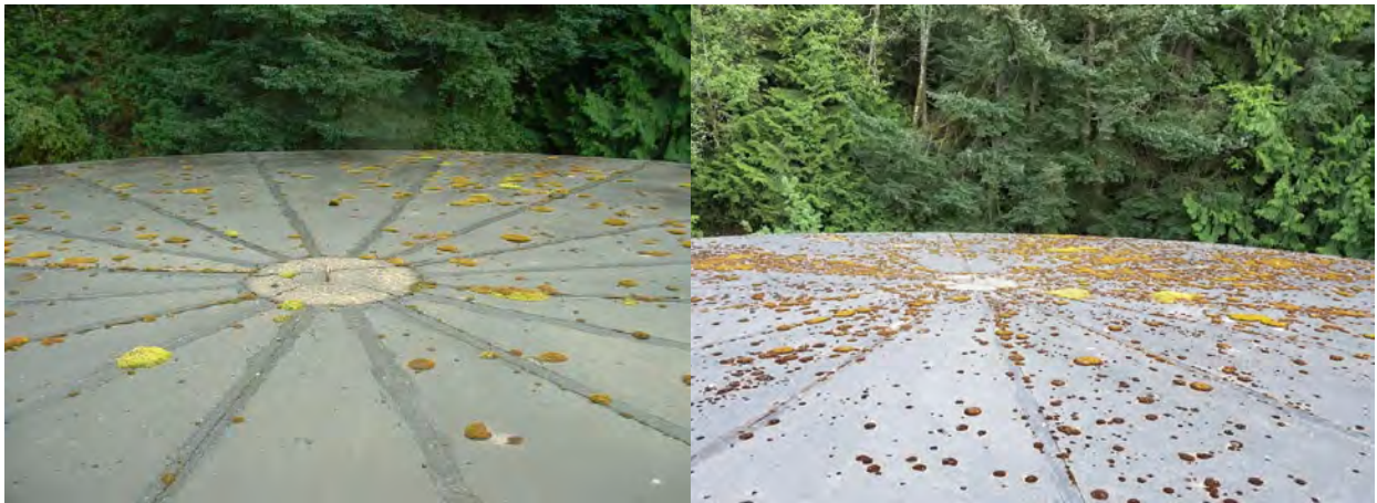
Figure A2.2.4: More green moss/vegetation growing on the roof, left picture from 2005, right picture from 2018
