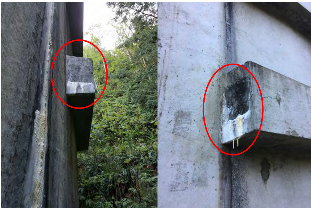
Figure A2.1.2: White efflorescence deposits at grout filled pockets on each end of the post tension buttress
