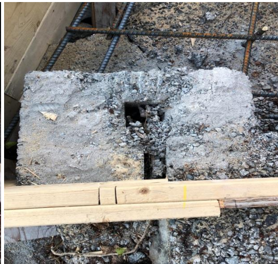
Figure #4: Vandalized/Cut off Corner Pillar on Lower Landing
