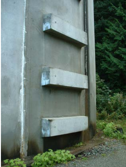
44. Anchor blocks for post-tensioned cables. South side of tank adjacent to large vertical leak (Water loss 4 liters per minute)
