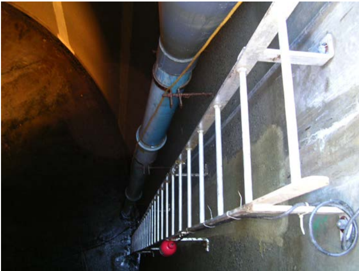
147. Access ladder and overflow pipe. Note corroded overflow pipe bracket supports
