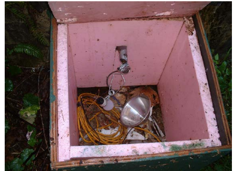
76. Insulated valve sensing line box
