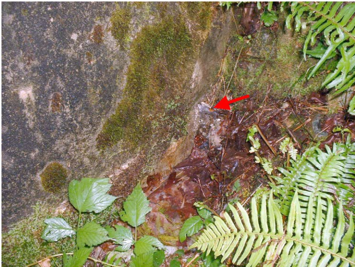
84. Hole at bottom of wall where water was observed to pouring out similar to water out of a tap
