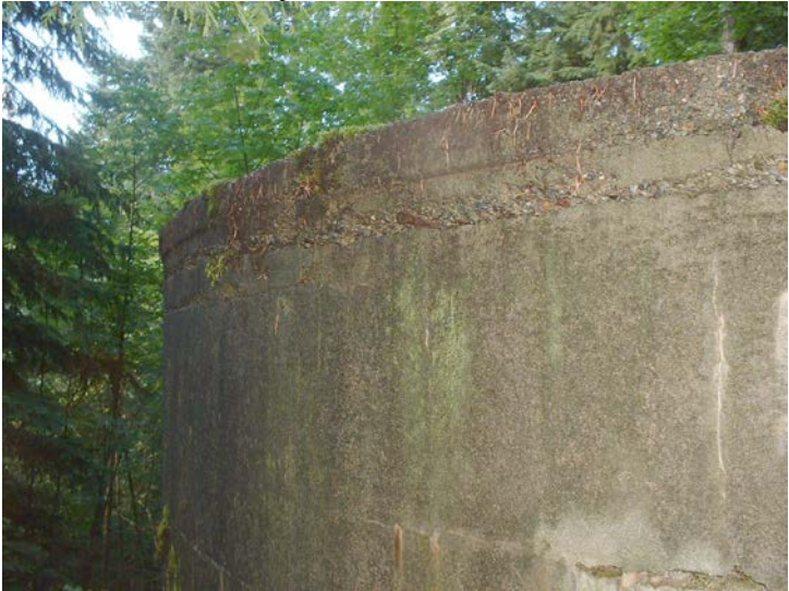
86. Horizontal crack at roof level on wall
