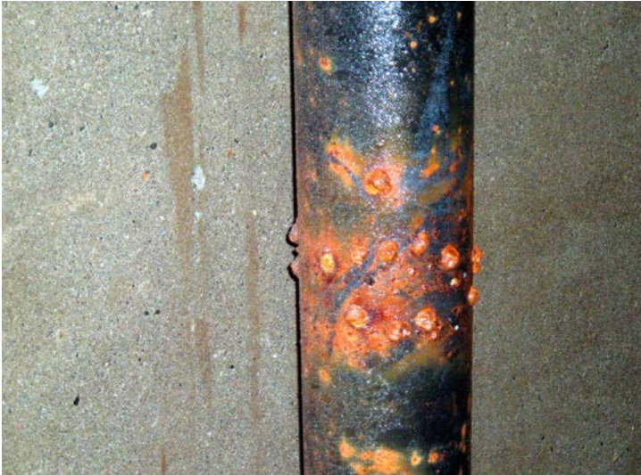
170. Corroded overflow pipe at mid height
