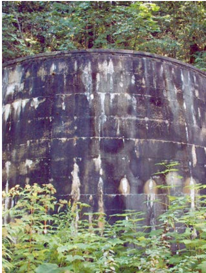
83. Vertical and transverse cracks
