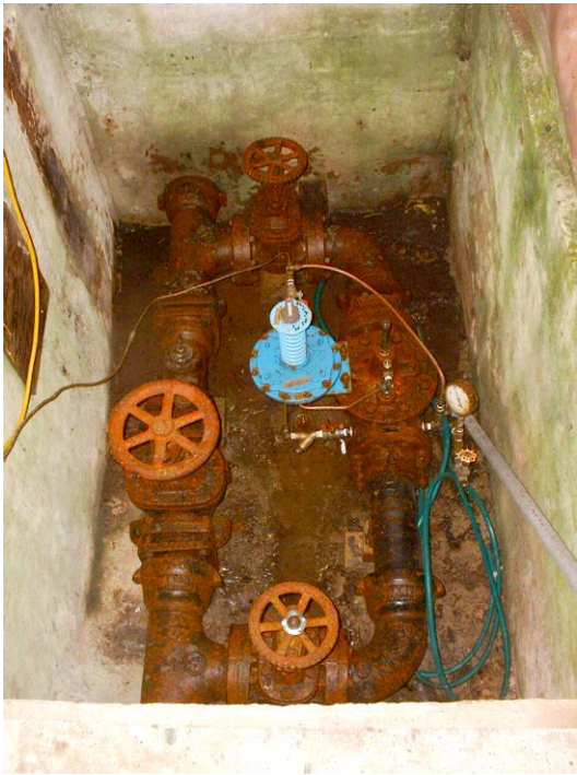
81. View of fill station valves
