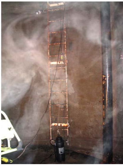
137. Corroded interior ladder
