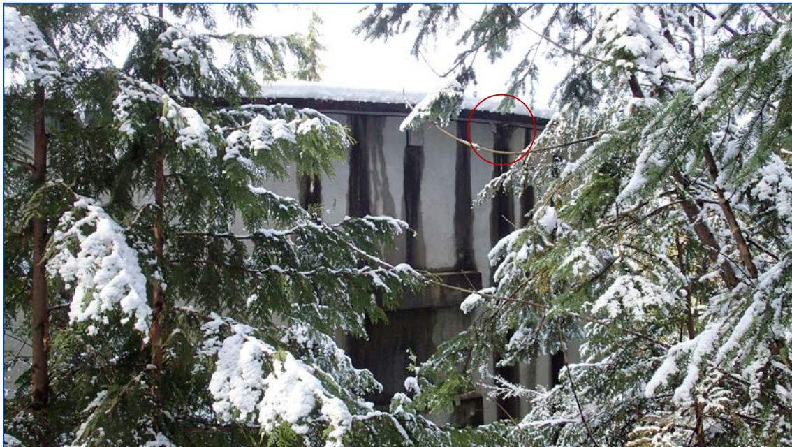
Photo 10: Presence of spall at the joint at the top of the reservoir wall.
