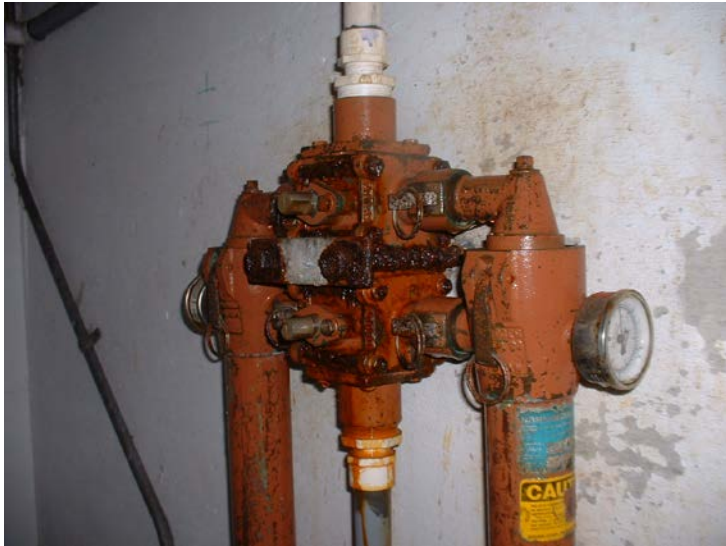
61. Mounting bolts corroded
