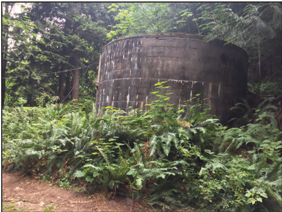
Figure 15: Phase V Tank, facing north.
