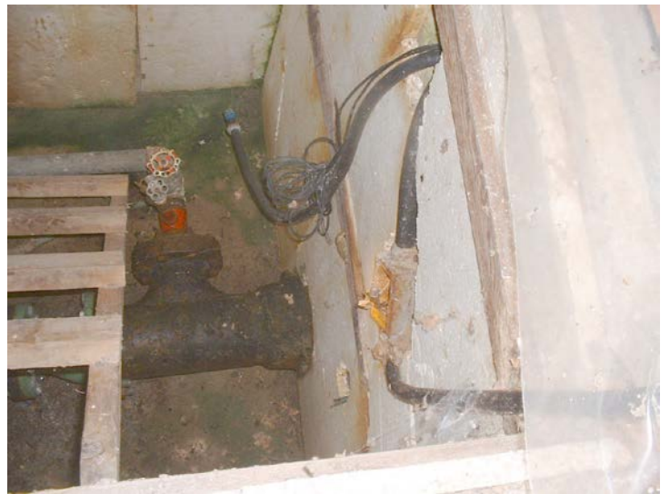
91. View of electrical box inside valve chamber
