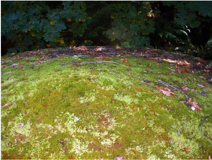
79. Vegetation and algae on roof
