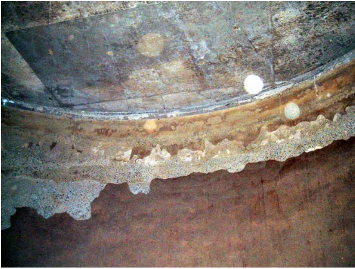
165. Cementitious coating material peeled off at top of interior wall.
