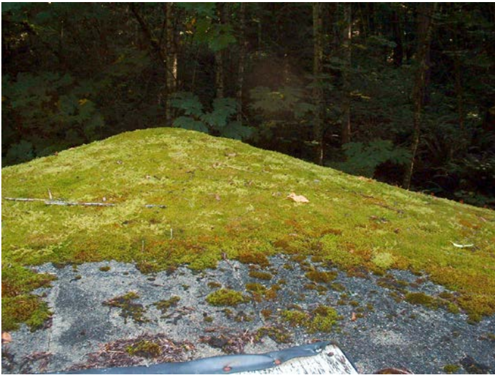
77. General photo of roof showing vegetation and algae
