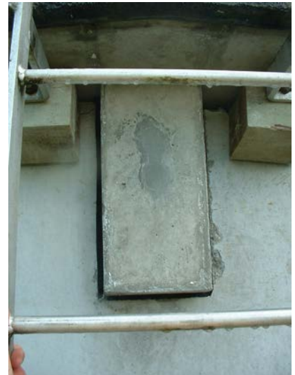
56. General view of concrete key locating roof concrete slab onto walls – NW side
