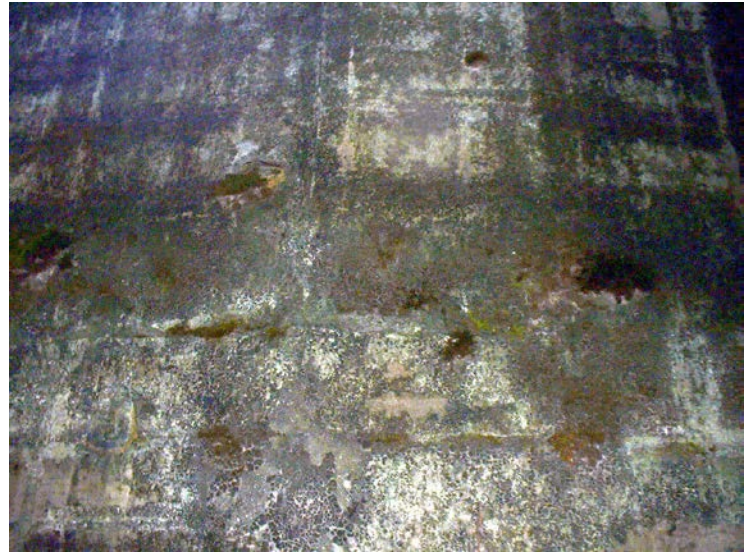
74. Algae growth on wall
