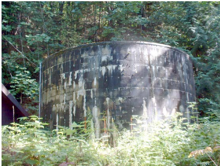
92. General view of cracking on wall
