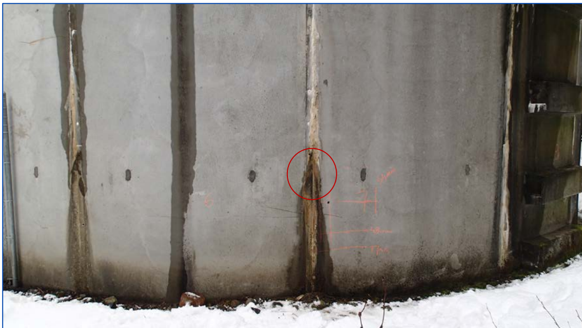
Photo 4: Leaking joints between the precast wall panels.
