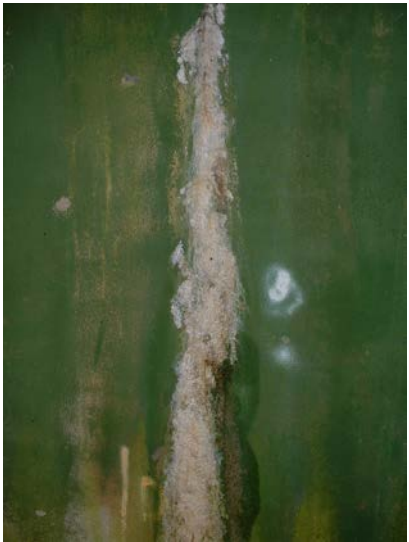
37. Efflorescence and corrosion stains at vertical crack
