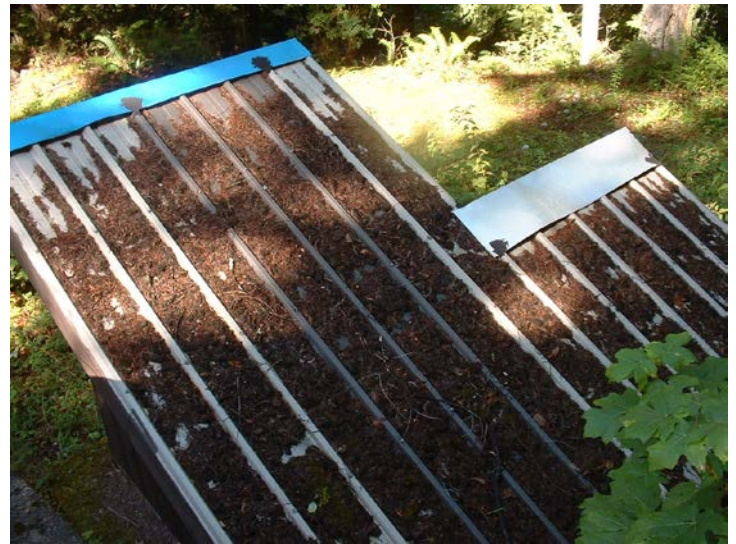
89. Debris on valve chamber roof
