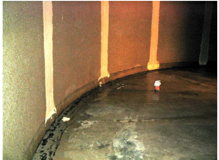
148. Rubberized type of coating material used along joint between the wall and base slab
