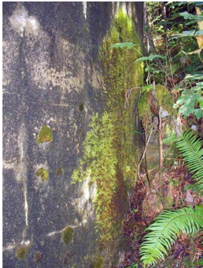
85. Algae growth on tank wall
