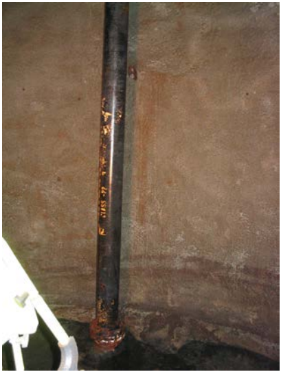
136. Overflow pipe slightly corroded
