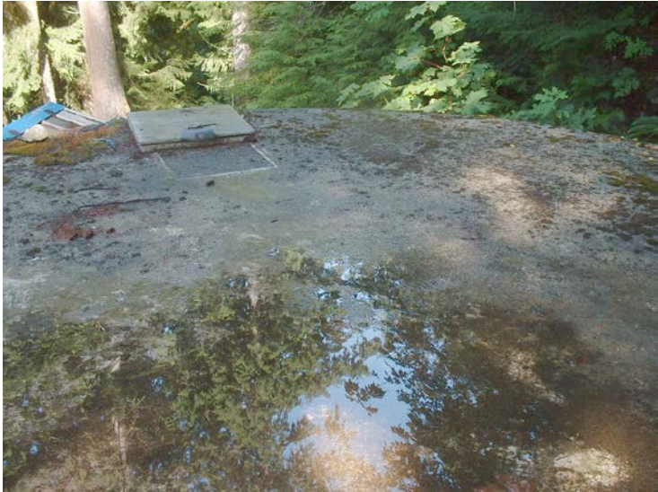
87. Water pooling on roof
