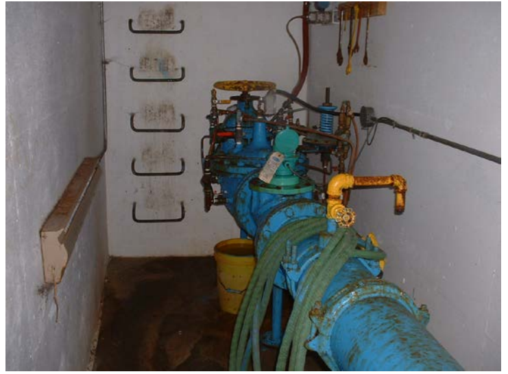
62. General view of inlet pipe in chlorination chamber
