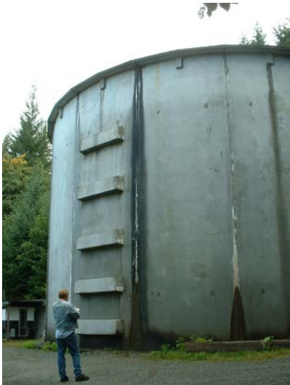
48. General view of anchor block adjacent to large leak
