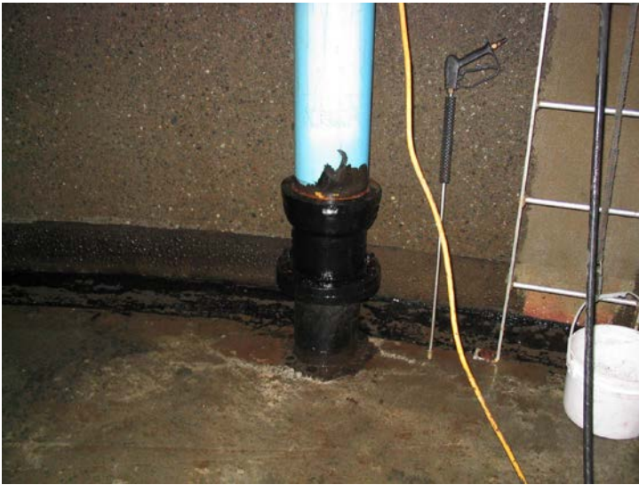
145. 200 pvc overflow pipe
