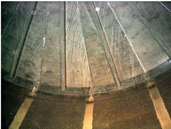
143. Note water leaking through roof panel joints
