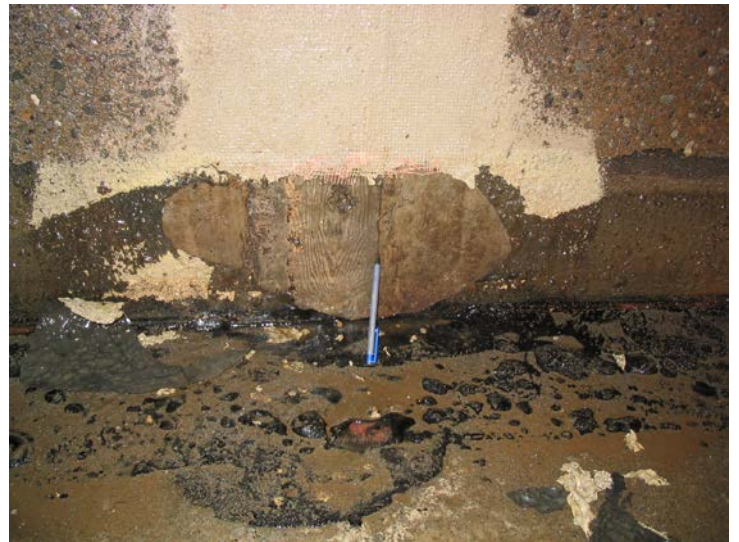
150. The rubberized material was easily pulled away from the wall and revealed vertical joints between wall panels. Water was seen to be leaking through this joint from the outside of the tank.
