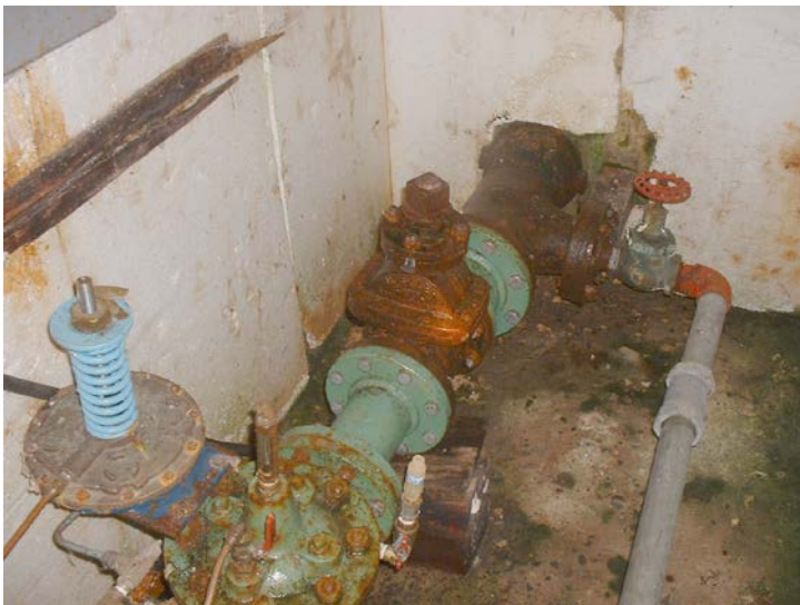
90. View of inlet pipe
