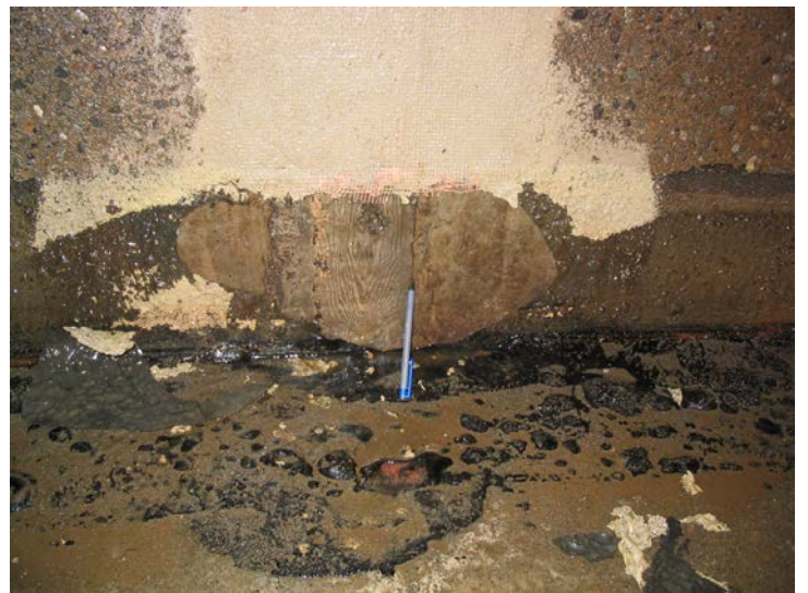
150. The rubberized material was easily pulled away from the wall and revealed vertical joints between wall panels. Water was seen to be leaking through this joint from the outside of the tank.
