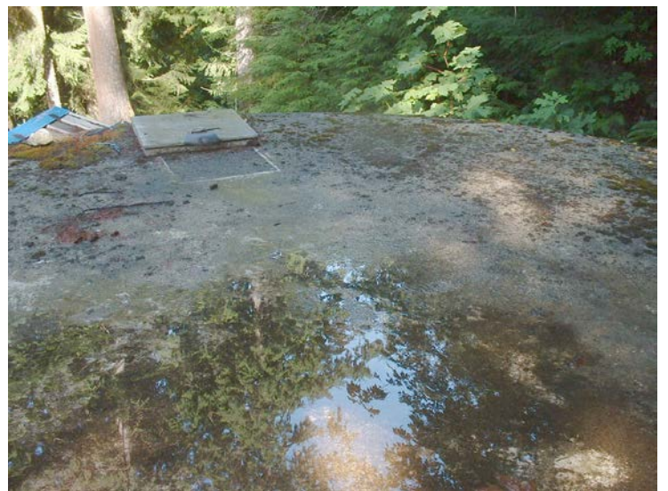
87. Water pooling on roof
