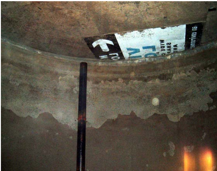
167. Missing anchorage at top of overflow pipe
