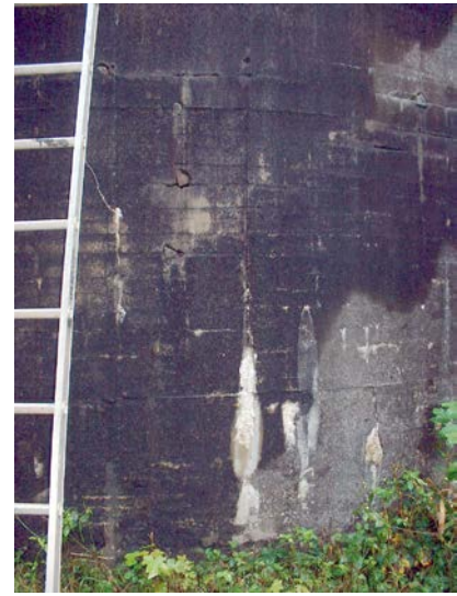
72. Vertical crack. Evidence of moisture and efflorescence
