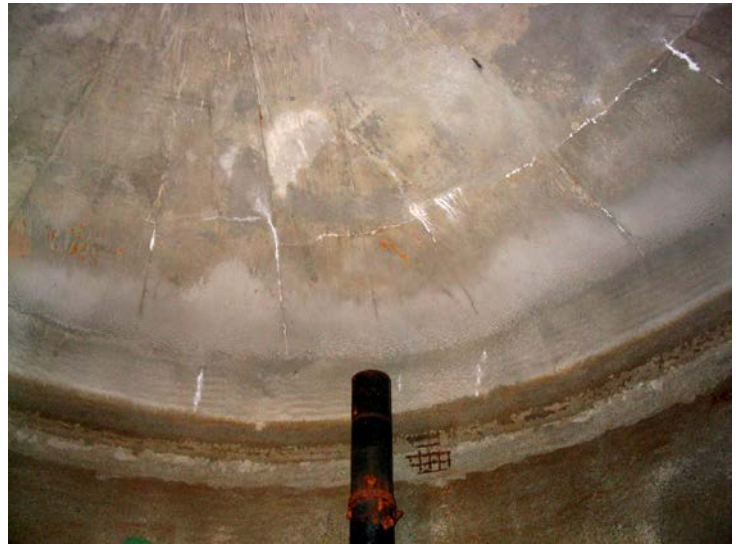
140. Underside of roof slab. Note cracks
