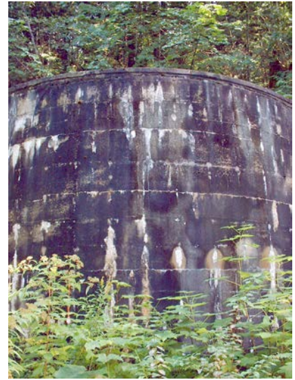
83. Vertical and transverse cracks
