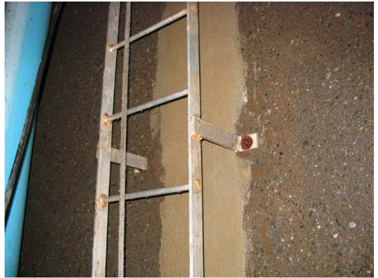
146. Corroded bolt at access ladder support inside of tank
