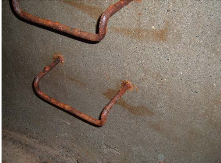
169. Corroded ladder rung
