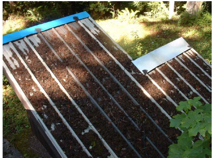
89. Debris on valve chamber roof
