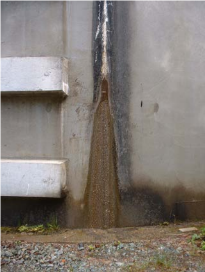
45. Large leak at wall panel junction
