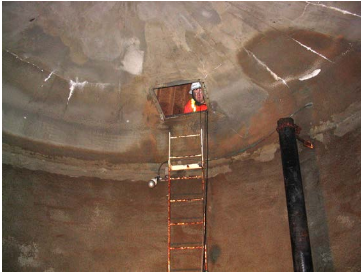
139. Underside of roof slab and interior ladder. Note cracks
