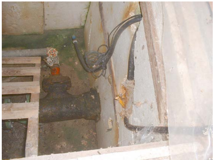
91. View of electrical box inside valve chamber
