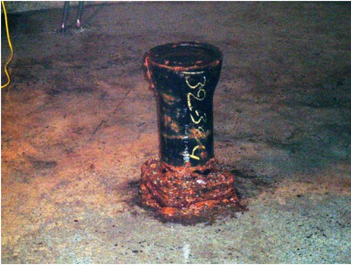
171. Corroded Outlet pipe on reservoir floor
