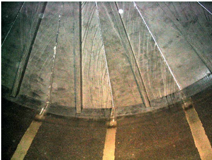
143. Note water leaking through roof panel joints
