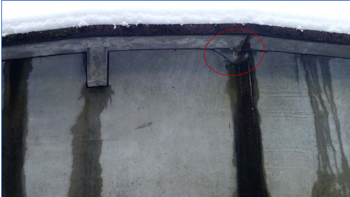
Photo 9: Close-up of Photo 8 showing a spall.
