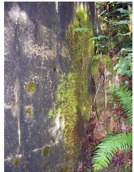
85. Algae growth on tank wall
