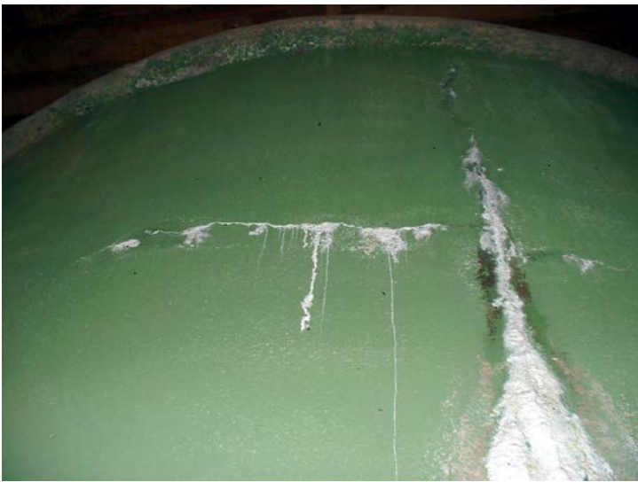
38. Horizontal and vertical cracks on tank western side
