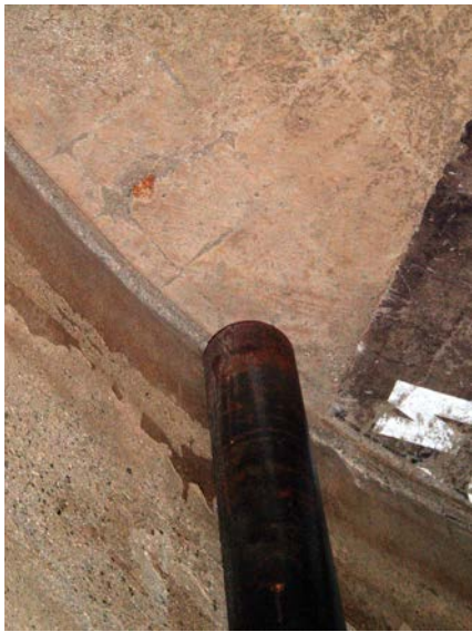
168. Missing anchorage at top of overflow pipe
