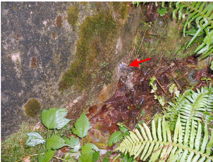
84. Hole at bottom of wall where water was observed to pouring out similar to water out of a tap
