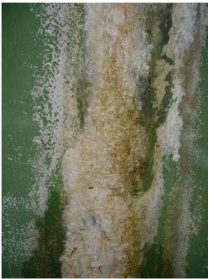
39. Efflorescence and corrosion staining at vertical crack
