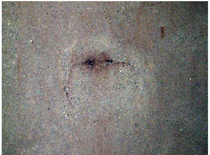
164. Cracked and delaminated concrete at east side of reservoir interior wall.
