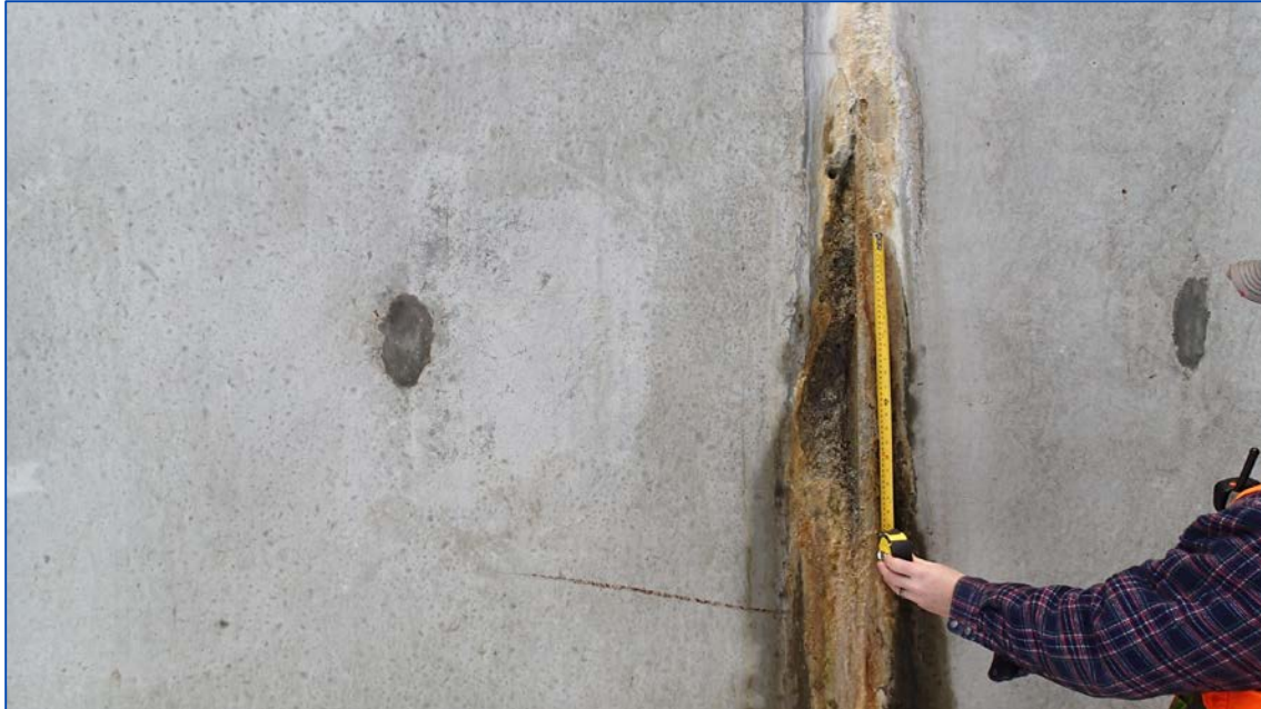
Photo 5: Close-up of Photo 4 showing deterioration of the joint.
