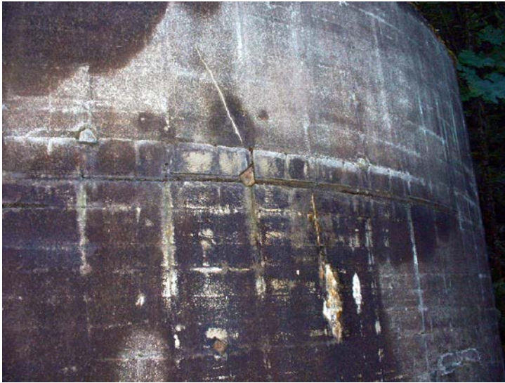
73. Evidence of honeycombed concrete at horizontal seam
