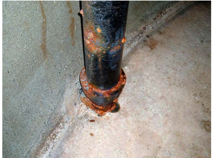
172. Corroded overflow pipe at bottom.
