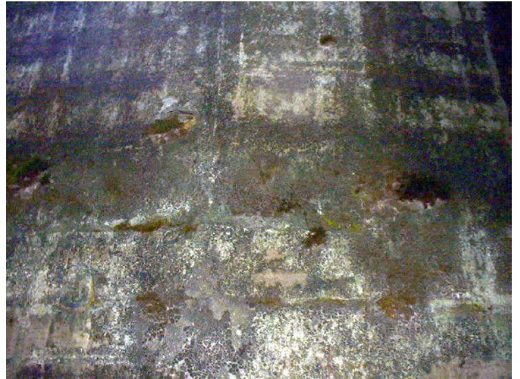
74. Algae growth on wall
