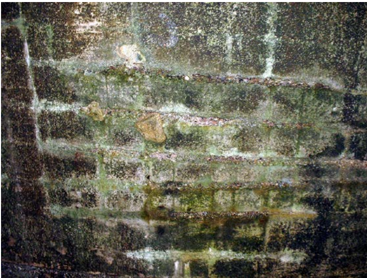
75. Honeycombed concrete along horizontal joints
