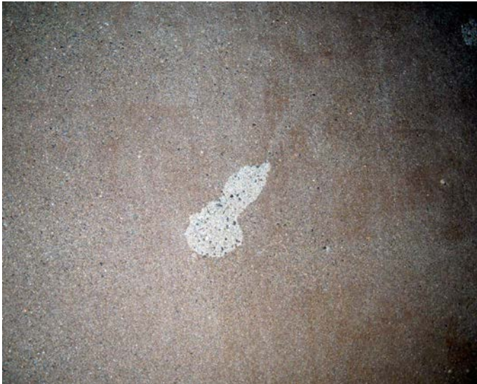
166. Spalling cementitious coating on interior wall.
