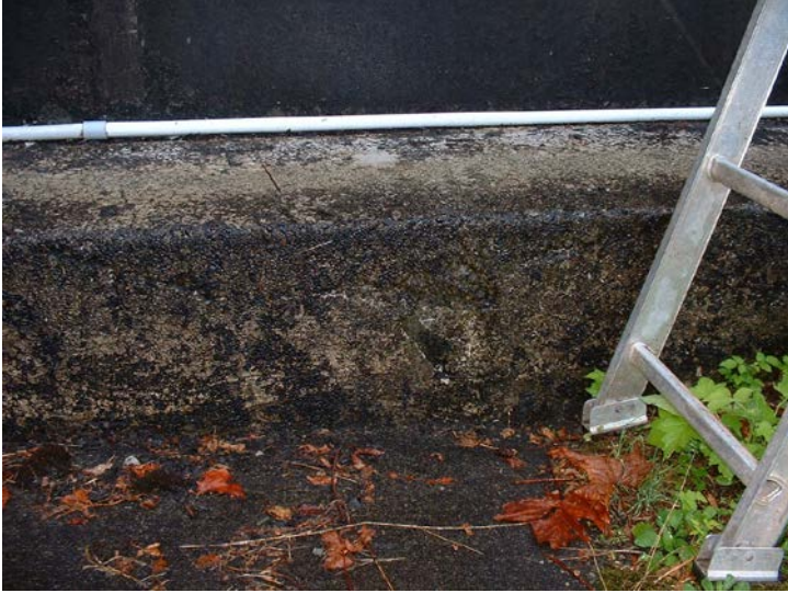
43. Honeycombing at wall foundation
