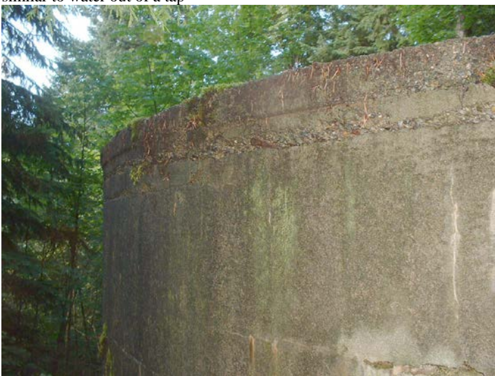
86. Horizontal crack at roof level on wall
