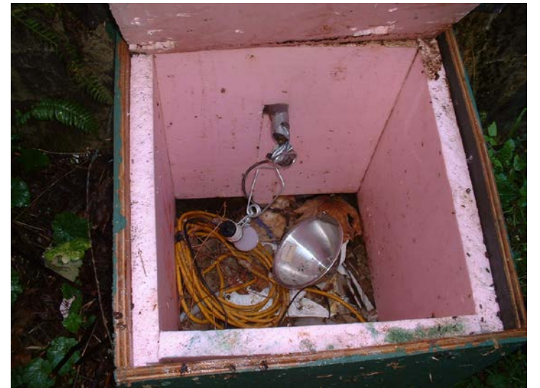
76. Insulated valve sensing line box
