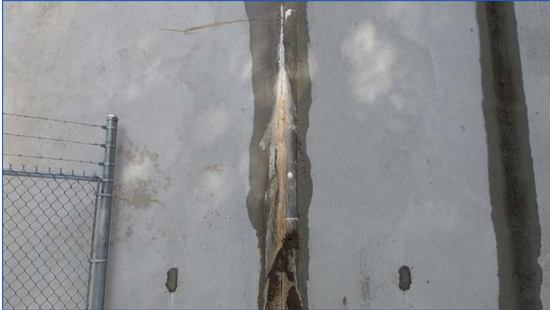
Photo 7: Presence of efflorescence at the joint between the precast wall panels.
