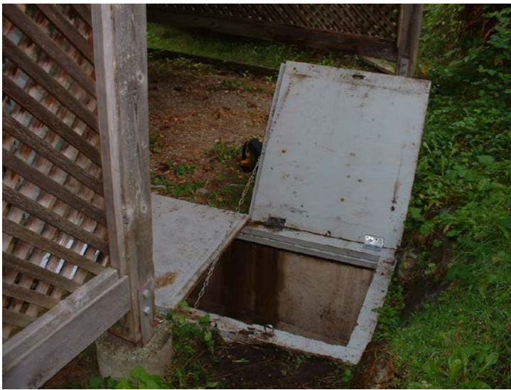
33. Open latch at valve chamber
