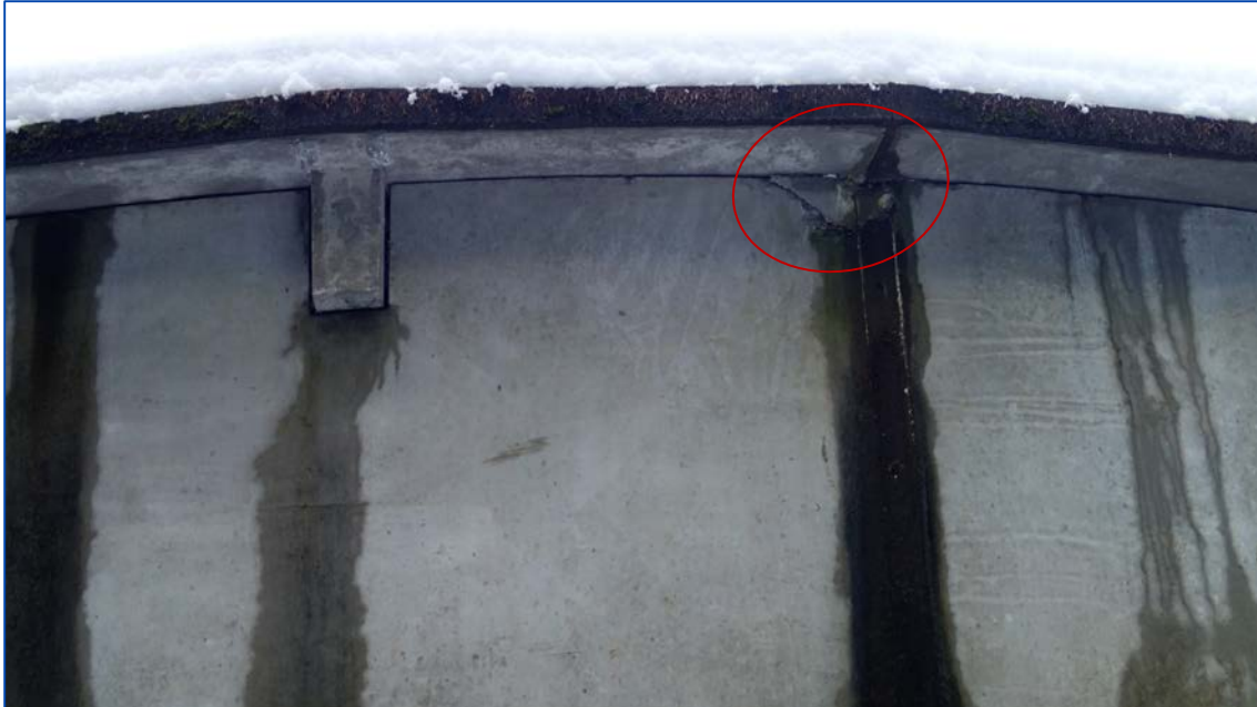
Photo 9: Close-up of Photo 8 showing a spall.
