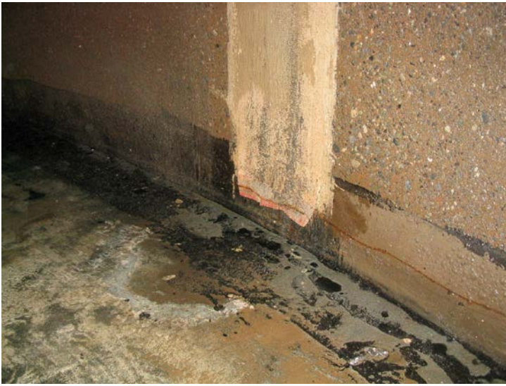
152. Evidence of general failure of sealing material along edge of wall and bottom slab and along the vertical joints in wall panels.
