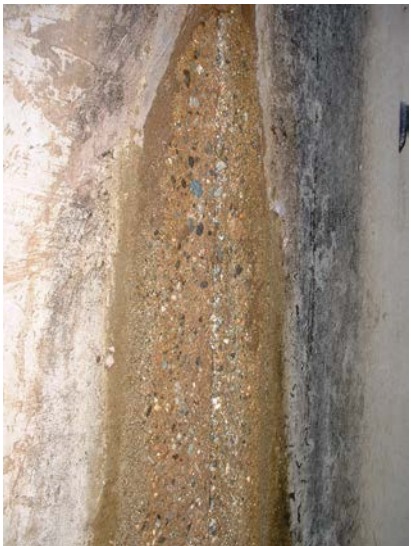
47. Close up of large leak
