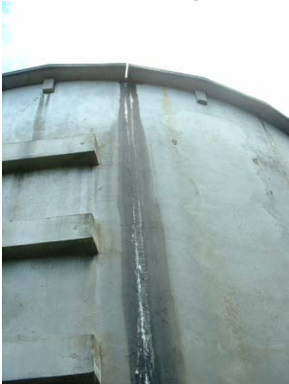
46. Upper half of tank at leak seam
