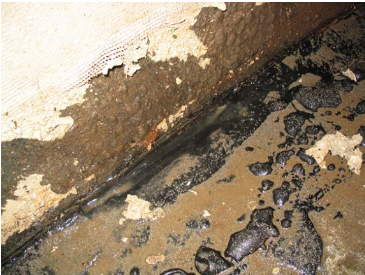
149. Evidence of failure (note air or water bubbles visible on the surface of the material) in the sealing material along joint between wall and base slab.
