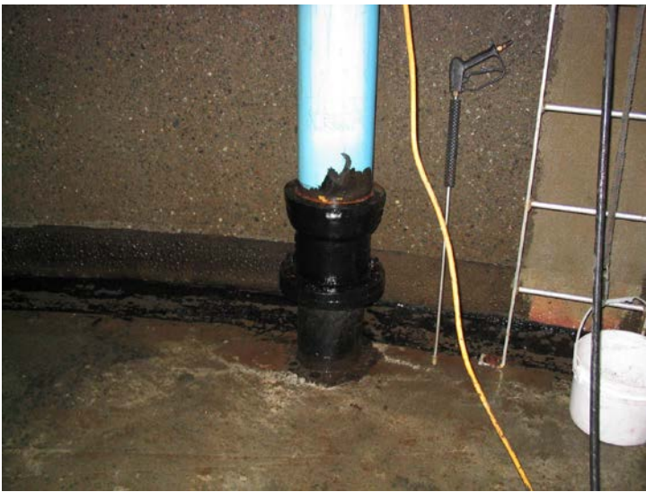
145. 200 pvc overflow pipe
