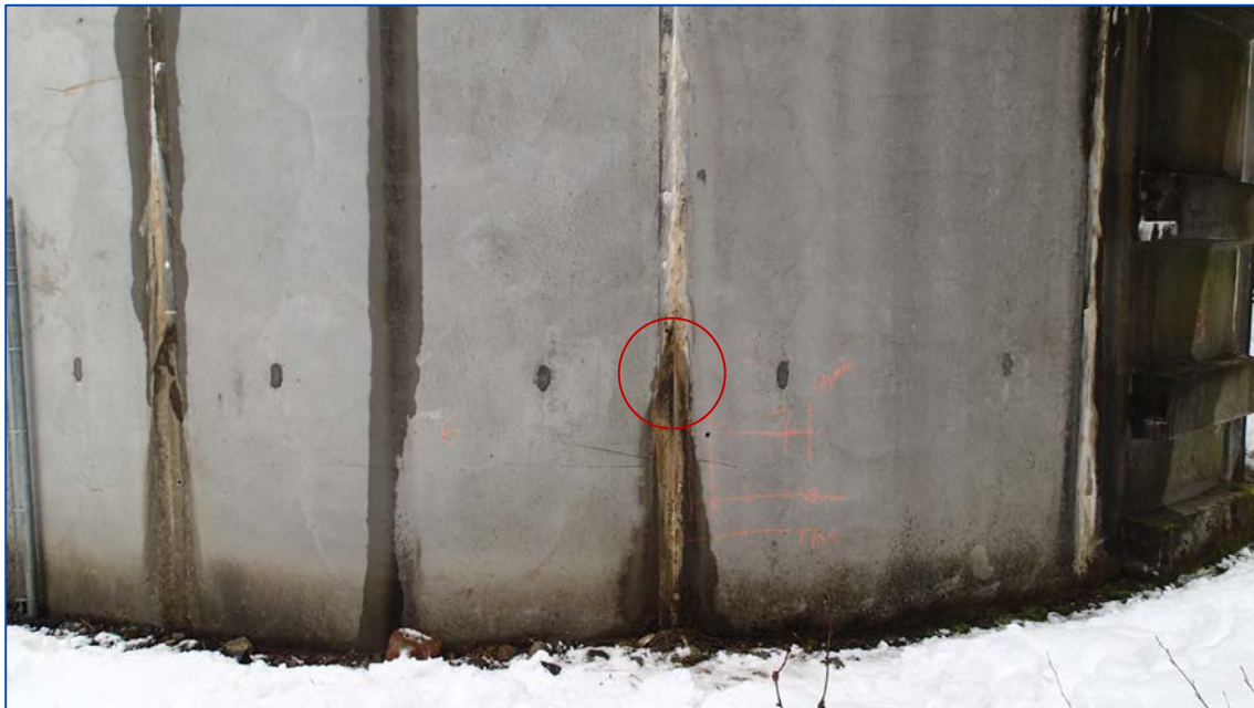
Photo 4: Leaking joints between the precast wall panels.
