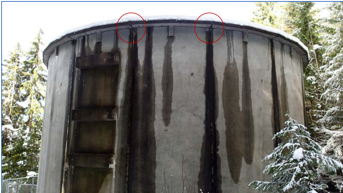
Photo 8: Spalls at the precast wall panel joints at the top of the reservoir wall.
