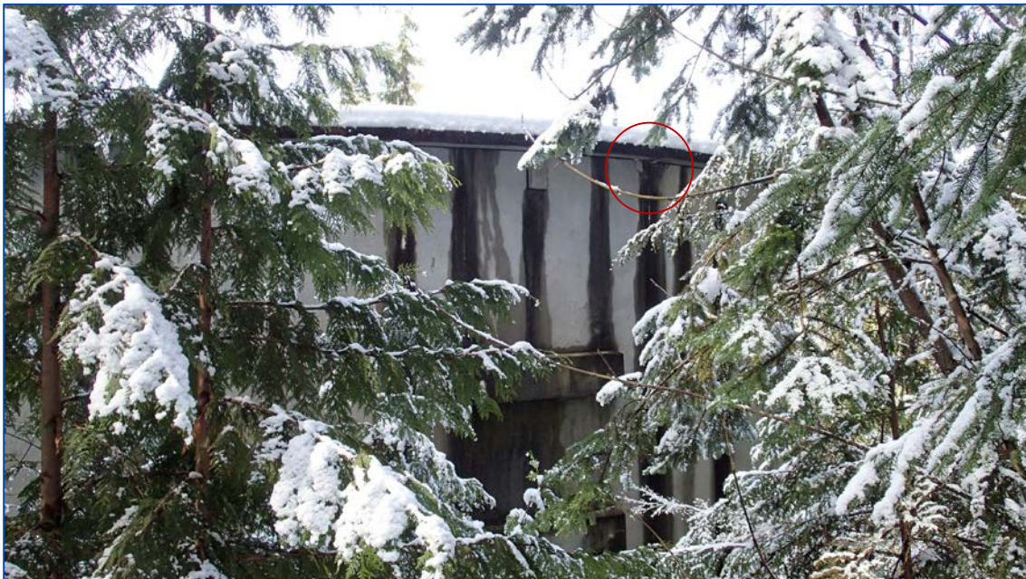
Photo 10: Presence of spall at the joint at the top of the reservoir wall.
