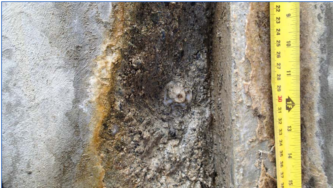
Photo 6: Close-up of Photo 5 showing deterioration of the joint.
