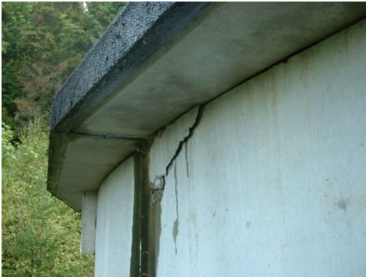
55. Spalling at top of wall – NW side
