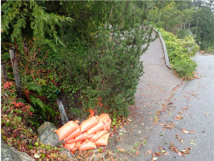
Photo 7. Lot 66 Kelvin Grove Way. Small Creek captured by drainage system undersized for full range of flows requires sand bagging to prevent overflow onto local road.
