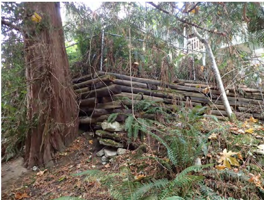
Photo 16. Substandard retaining walls represent a slope hazard.
