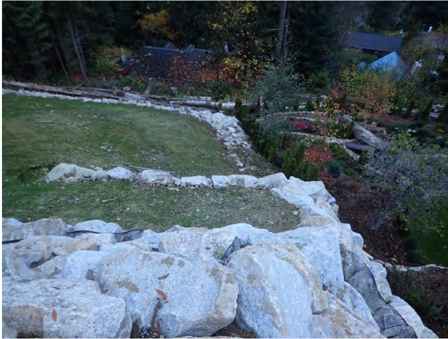
Photo 15. Stacked rock wall in steep terrain using geotextile to tie back into slope.
