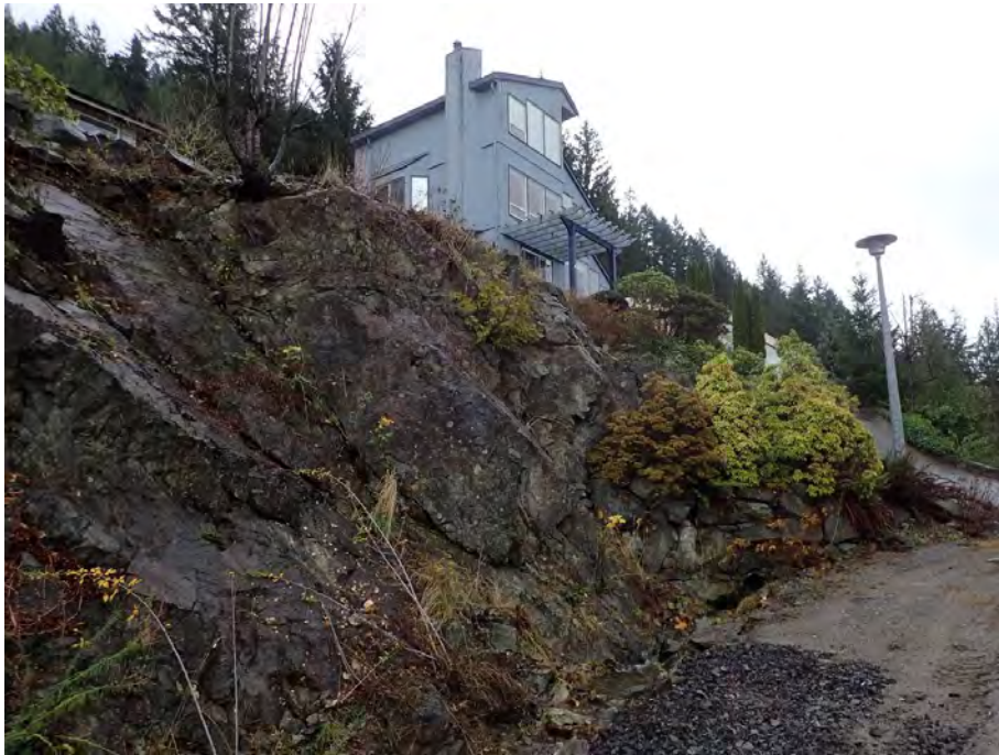
Photo 9. Unfavourable jointing in road cut, Lot 85 Kelvin Grove Way.
