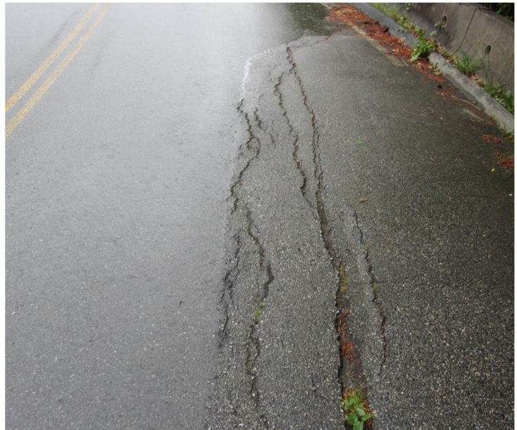
Figure 5-2: Photo of Edge Cracking
